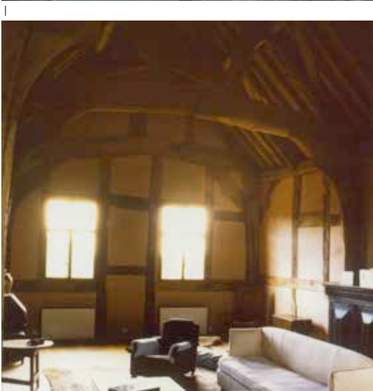
2 Repair and conversion of 14th century timber framed building and 17th century house to form holiday accommodation.
